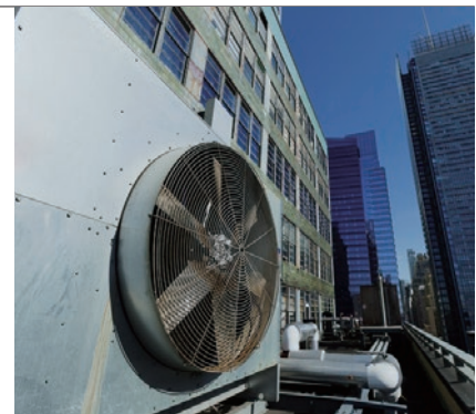
Air conditioning system
