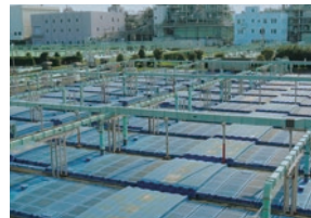
Water treatment plant
